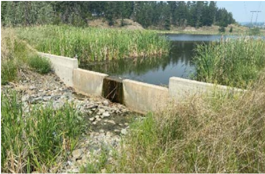
CONCRETE WEIR (FIXED)
